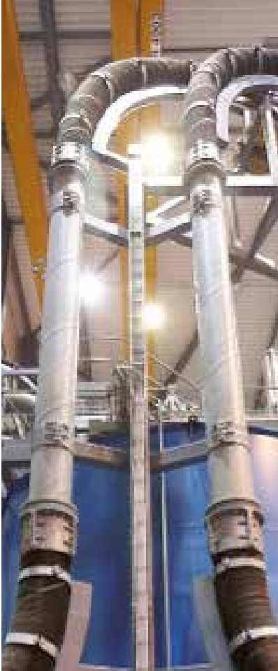
Picture 1: Material handling hose and rubber lined steel pipe
