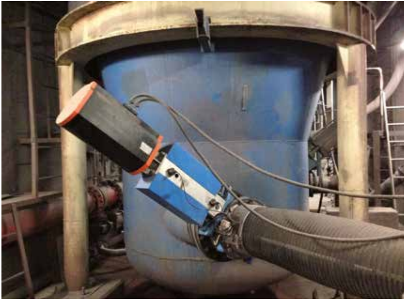
Sump tank with shut off valve
