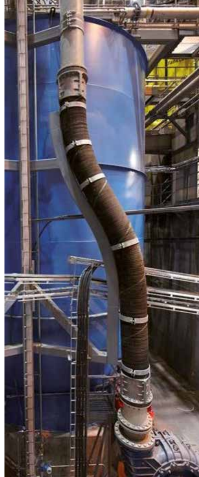
Picture 2: Material handling hose with support beam and clamps
