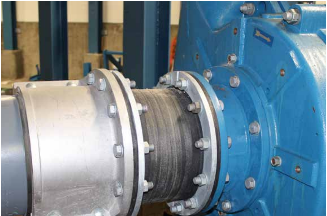
Picture 5: Rubber lined steel pipe and compensator
