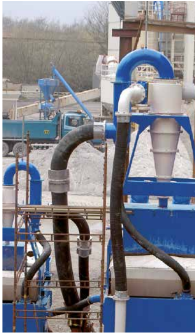
Picture 4: Material handling hose with 3x90 degree bend
