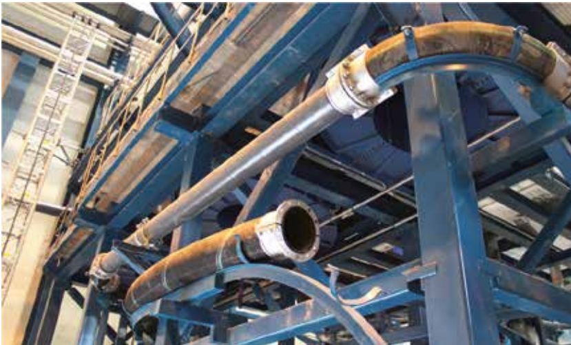
Picture 3: Material handling hose, rubber lined steel pipe, 3xD 90 Degree bend and support clamps
